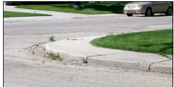
Absent curb cut
