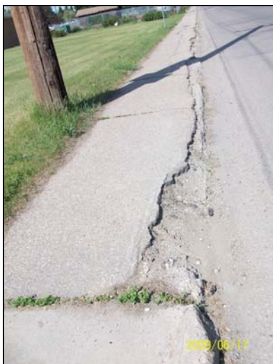
Poor sidewalk condition
